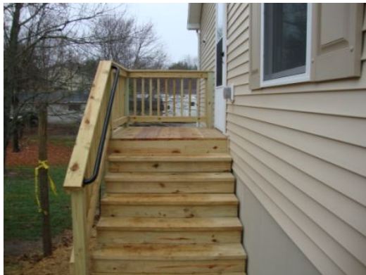
Handrail along guardrail
