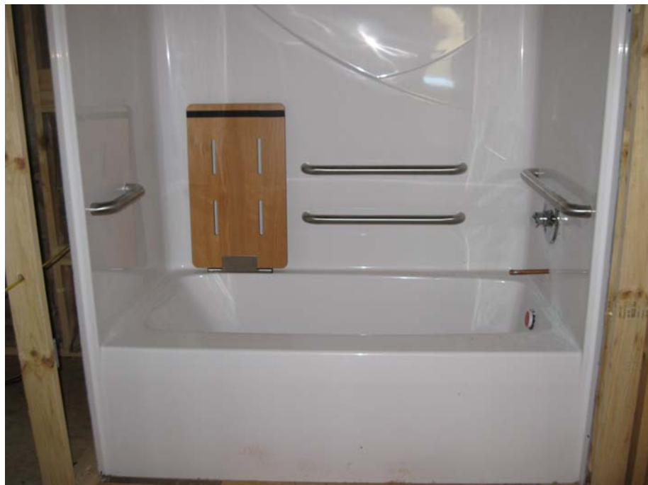
ADA Compliant Bathtub
