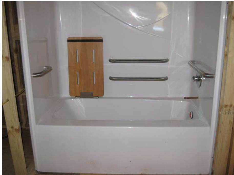
ADA Compliant Bathtub
