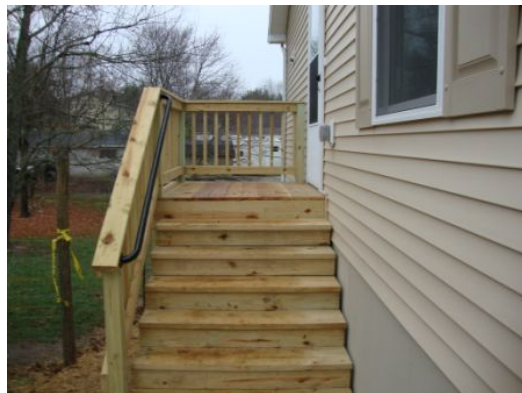
Handrail along guardrail
