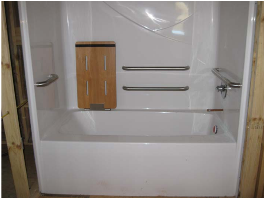
ADA Compliant Bathtub
