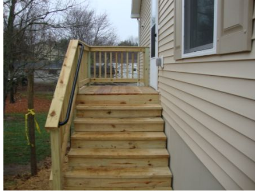
Handrail along guardrail
